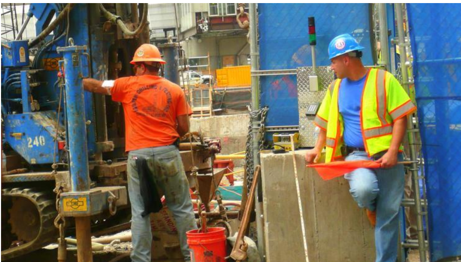
Two construction workers at a New York City work site. (Photo by Sheila.) SHEILA | CC-LICENSED
